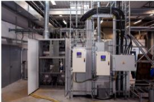
Electrolyser 30 Nm 3 /h
